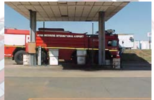
Airfield-fuelling station in Johannesburg/ South Africa, equipped with the TA 2331 from Hectronic.
